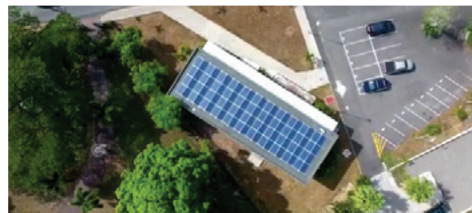
The Centre for Advanced Research in Renewable Energy at the University of the West Indies.
